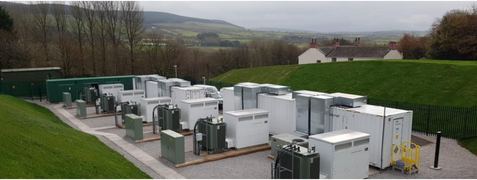
Photograph of the typical layout of a Battery Storage Facility.
